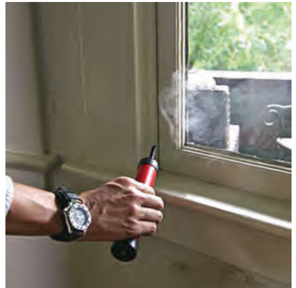
A smoke puffer is used around this window during the blower door test to make air leaks more visible to the technician and homeowner.
