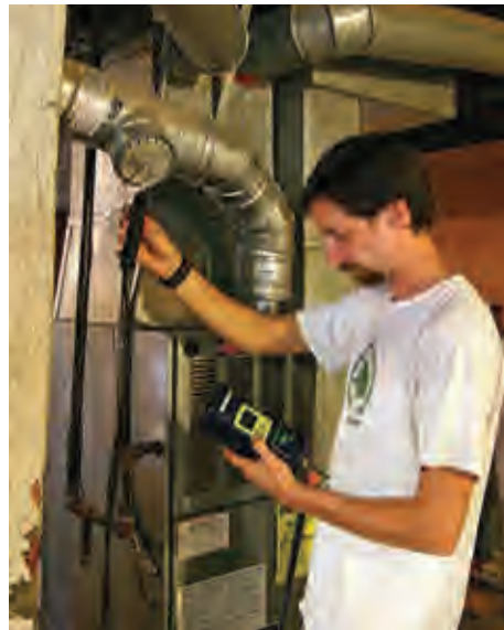
A combustion analyzer is used to look at carbon monoxide output and combustion efficiency of a gas furnace.
