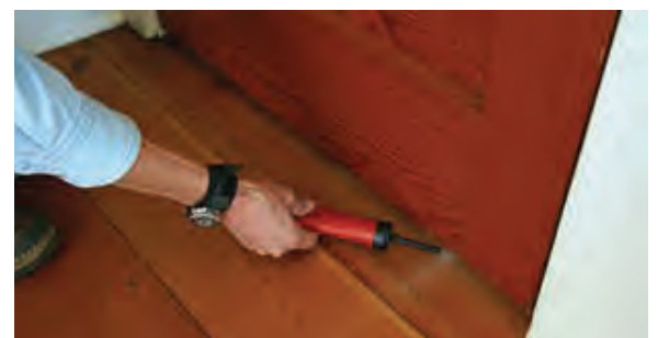
Door leading to the basement without a threshold gasket proves to be a large air leak in this home.
